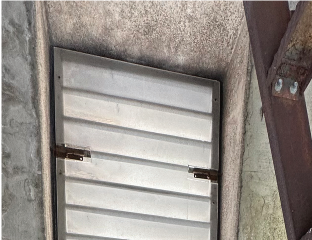
Bell Tower louvers are typically slatted wood screens held in place by throw bolts. They do not resist weather.
