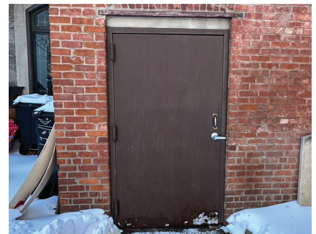
The Parish Hall first floor exit door is mismatched to the historic character of the building, and has deteriorated.
