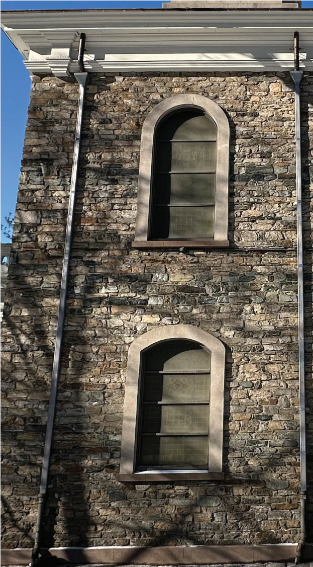
All four walls of the Church are made of mass stone masonry, and are in good condition.
