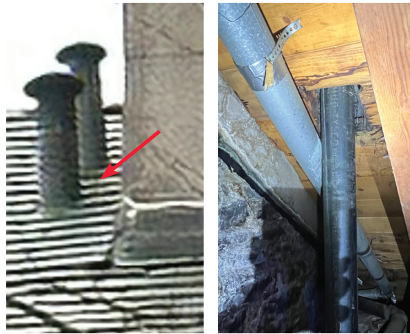
A02 - REPAIR FAILED ROOF VENT FLASHING
