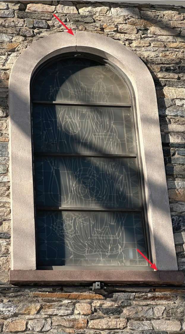
Surrounds have typically cracked at the top of the arch, and horizontally cracked at sills, at both nave and mezzanine level windows.
