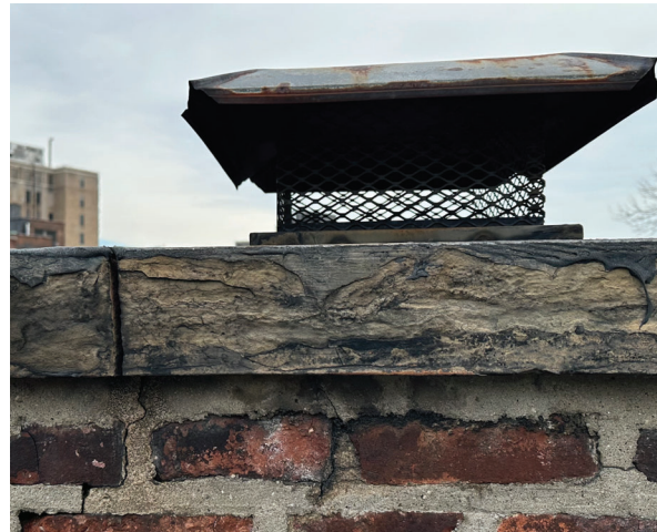
A15-3 - INSTALL WEATHER-RESISTANT CHIMNEY
