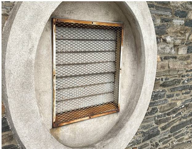
The Church attic vent louver at the north pediment does not reliably resist weather, has a rusted frame, and is mismatched to the style of other church louvers.
