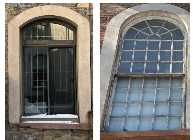
A16-1 - REPAIR OR REPLACE DETERIORATED WINDOWS
