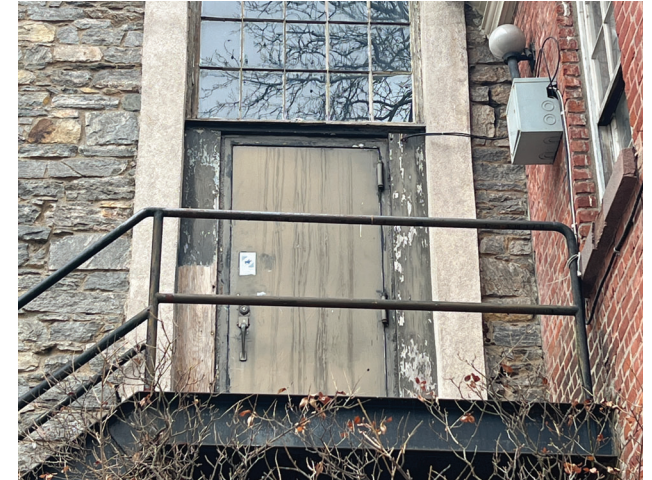
The Parish Hall emergency exit door from the second floor is out of place as a flat metal panel in a window wall. Its plywood frame has failed.
