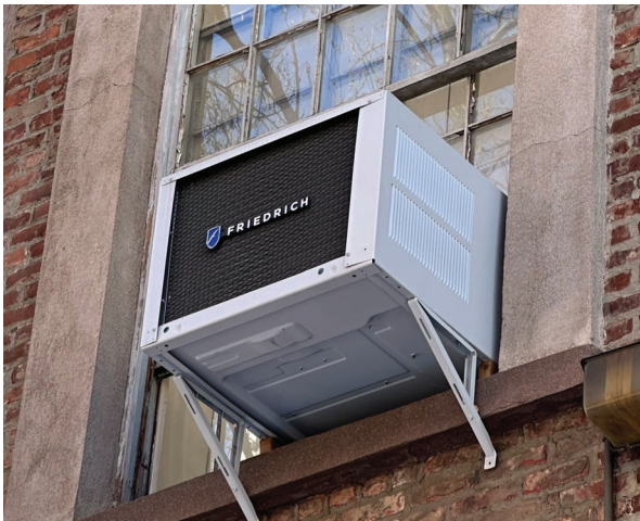
A04 - PROVIDE WEATHER SEALS AT A/Cs
